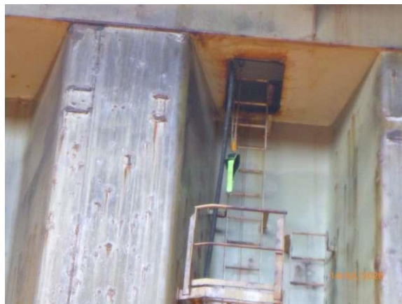
Figure 5: A safety belt with shock absorber and lanyard attached to a rope which is fixed on a hatch opening; the seafarer removed the safety belt to move down the fixed vertical ladder, before falling from a height of approximately 8 m to the cargo hold bottom and sustaining fatal injuries
